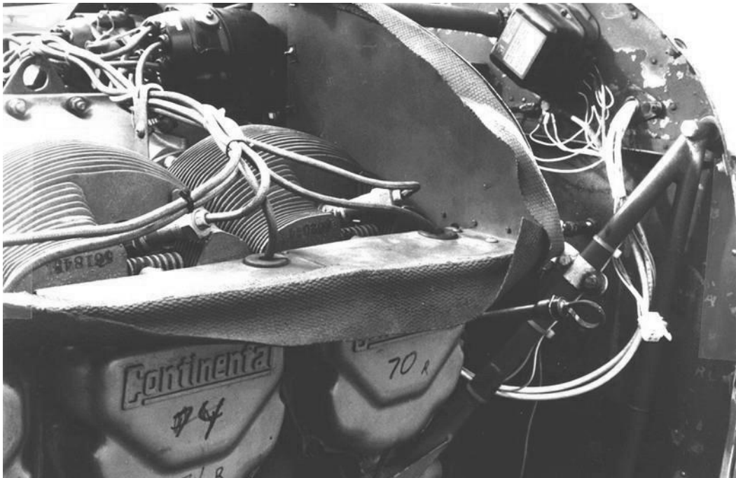
Figure 6-75. Improperly Positioned Baffle Seals
